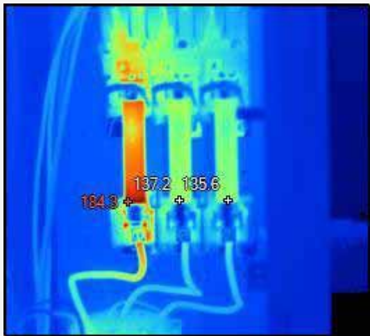
COMMON COMMERCIAL USE FOR COLOUR HANDHELD THERMAL IMAGER, DETECTING OVERHEATING IN ELECTRICAL SYSTEMS.
