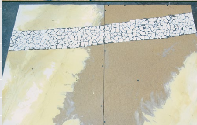
Step 5) Gently blow the sand away with a can of compressed air. The sand should be left neatly filling the gaps.
