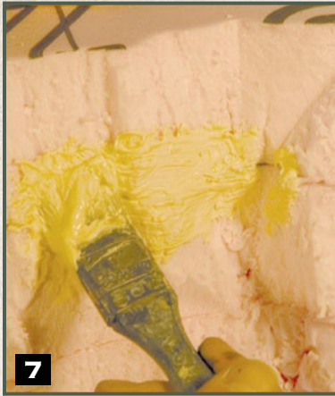
7 Step 7.) I know what you're thinking: Look at that huge seam. Just liberally spackle over the seams, making sure to thoroughly fill the gaps.
