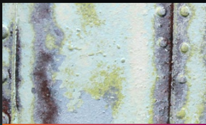
close up of the peeling white paint
