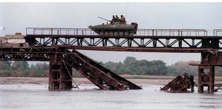
A BMP-B crosses the upper Elbe River east of Praha on a bridge repaired by troops of the 91 st Pontoon Regiment, April 1999.
